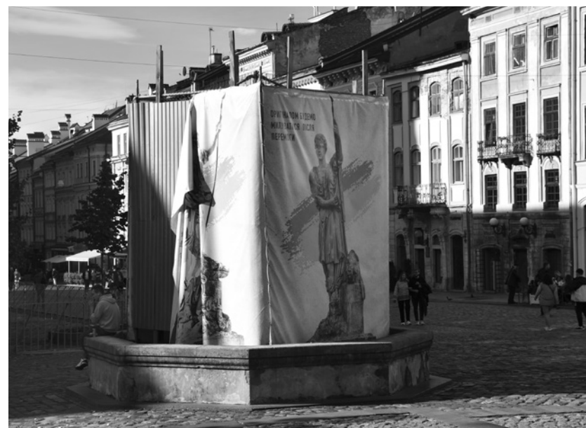
▣ Statue of Neptune at the Lviv Market Square secured with scaffoldings and corrugated metal sheets, January 2023
